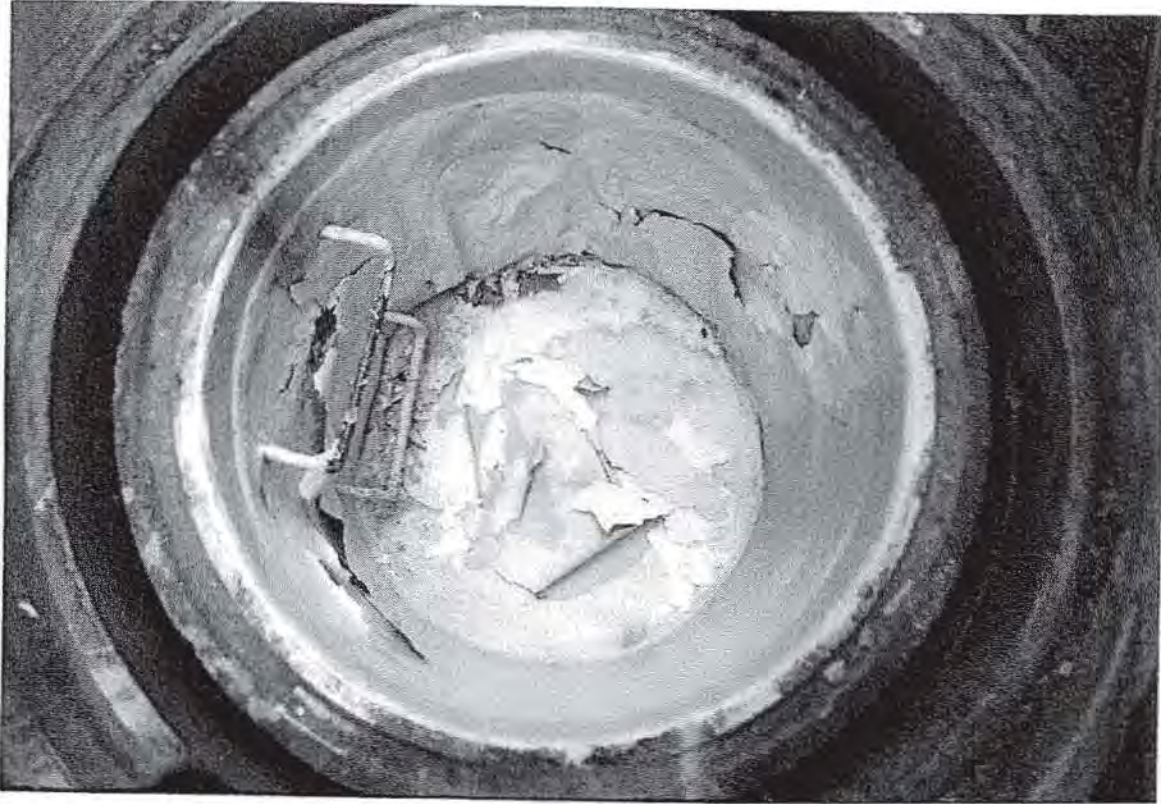
Figure 7. Epoxy coating failure.
