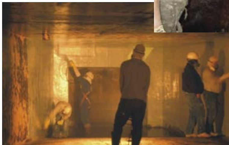
A crew from F&L Concrete Services spray-applies the new coating to protect concrete surfaces from corrosion.
